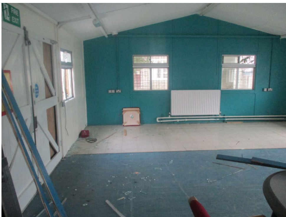
Damaged education area after recent incident of disorder
