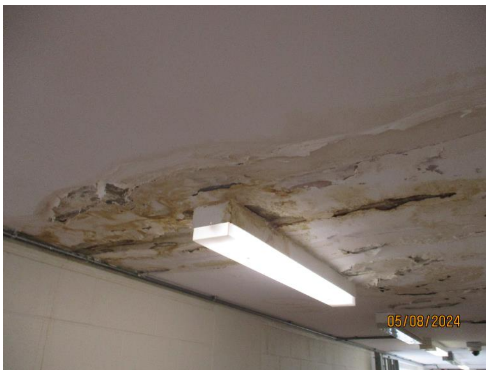
Secure corridor damage
