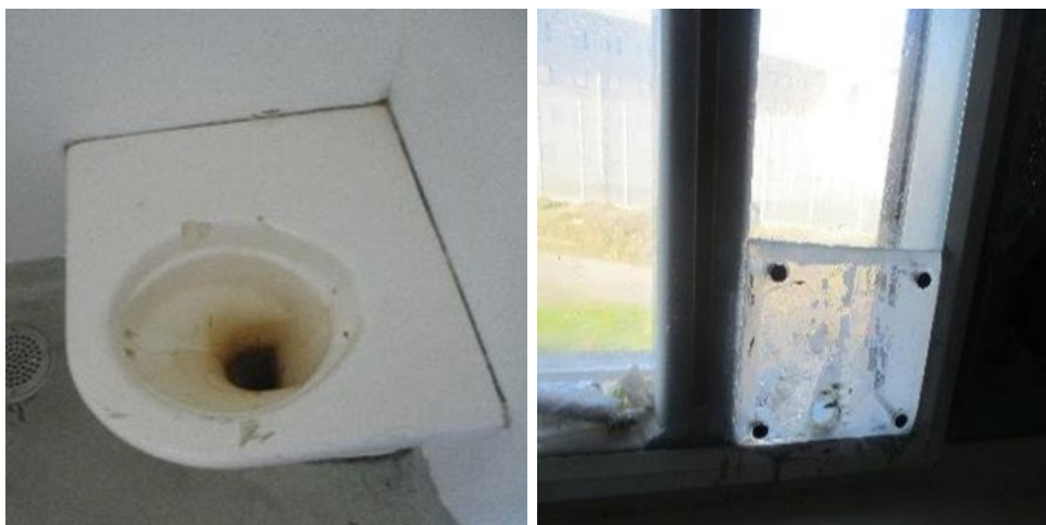
Segregation unit toilet (left) and repaired window in segregation unit
