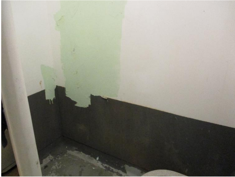
Typical in-cell shower with peeling paint
