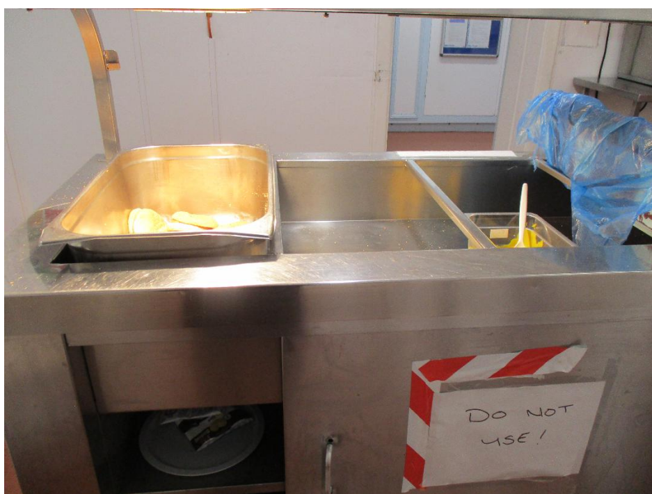
HMP Usk broken kitchen equipment
