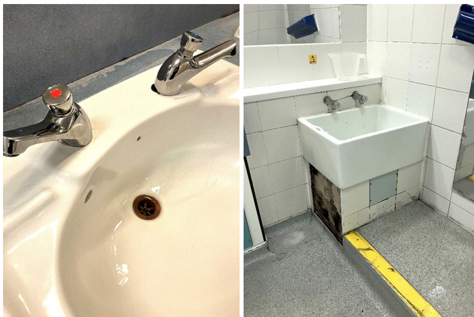
Broken taps in bathroom (left), and broken and missing tiles in bathroom (right)
