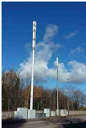
Dedicated Radio Mast
