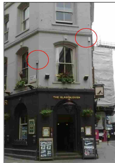
2 micro cells on side of building
